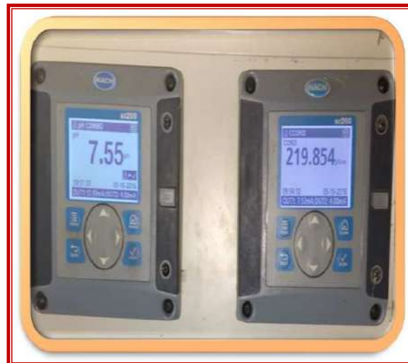
Effluent Quality Monitoring System
