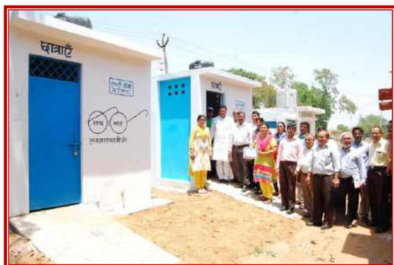
Toilet Constructed by NTPC under Swachh Bharat Abhiyan
