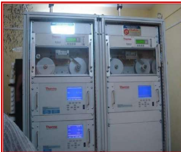
Continuous Ambient Air Quality Monitoring System
