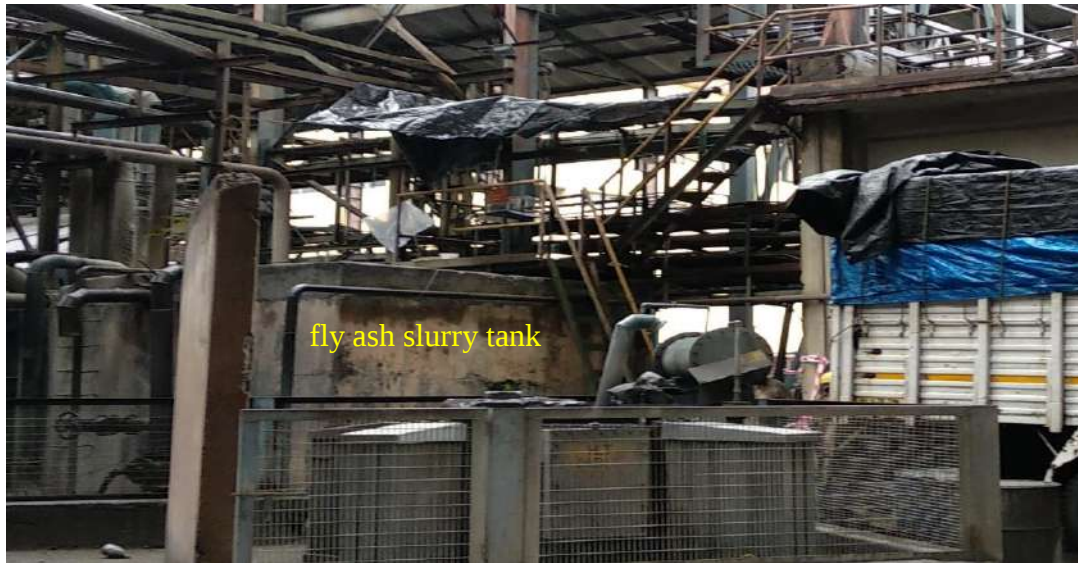
Figure 4: fly ash slurry tank inside the plant
