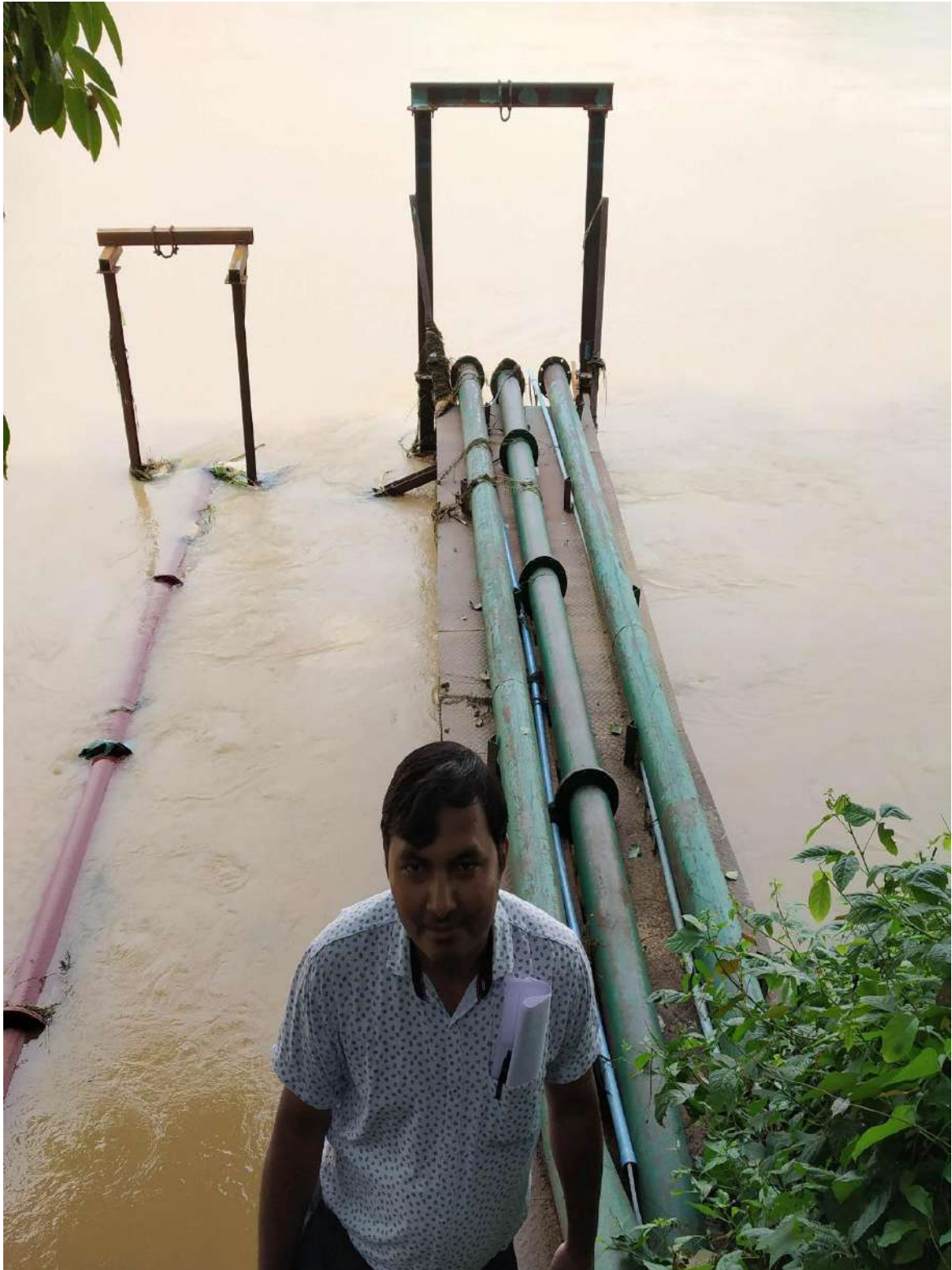
Fig. 3.3 Intake of P.H. Division, Angul (Water Supply to Talcher town)
