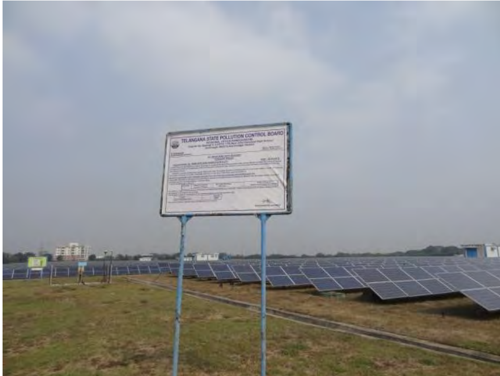
Figure -3 NTPC Solar power plant
