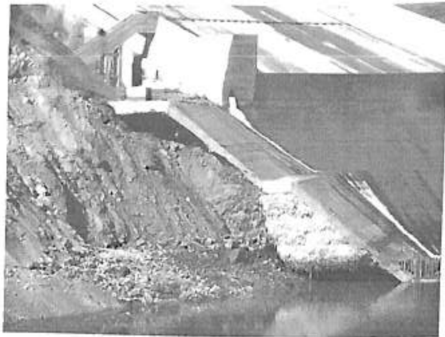
Photograph showing cavities below cladding on the right bank
