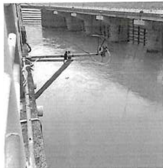
Automatic Water Level Recorder
