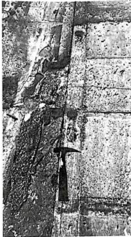
Photo 2 : Typical Longitudinal Dilation joint which is smooth and straight and doesn't show signs of cracking
