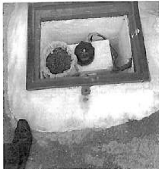
Strong Motion Accelerograph near the Right Abutment on the top of Dam
