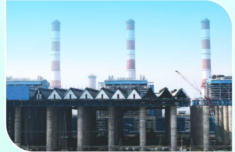
Air Cooled- Condenser at NTPC North- Karanpura
