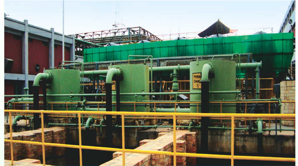
Neutralization Pit at DM Plant
