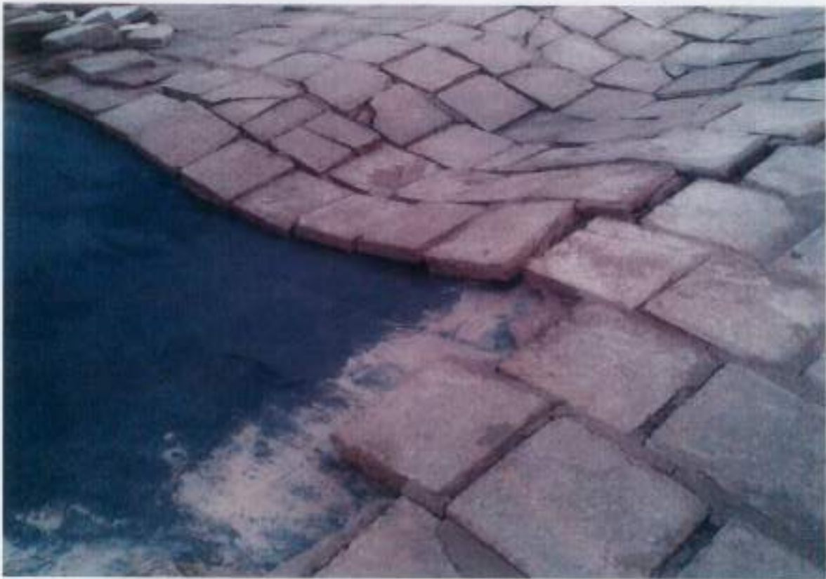
Heavy depression on upstream slope
