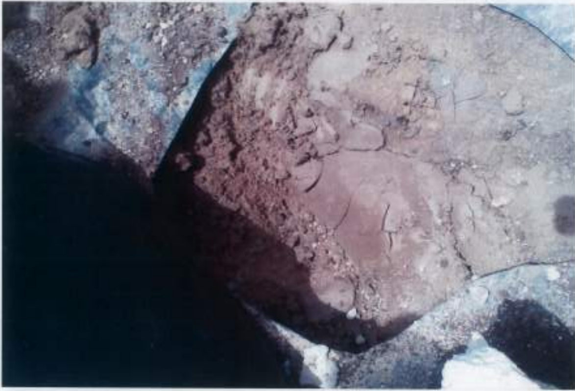
Loose soil under the HDPE layer on upstream toe
