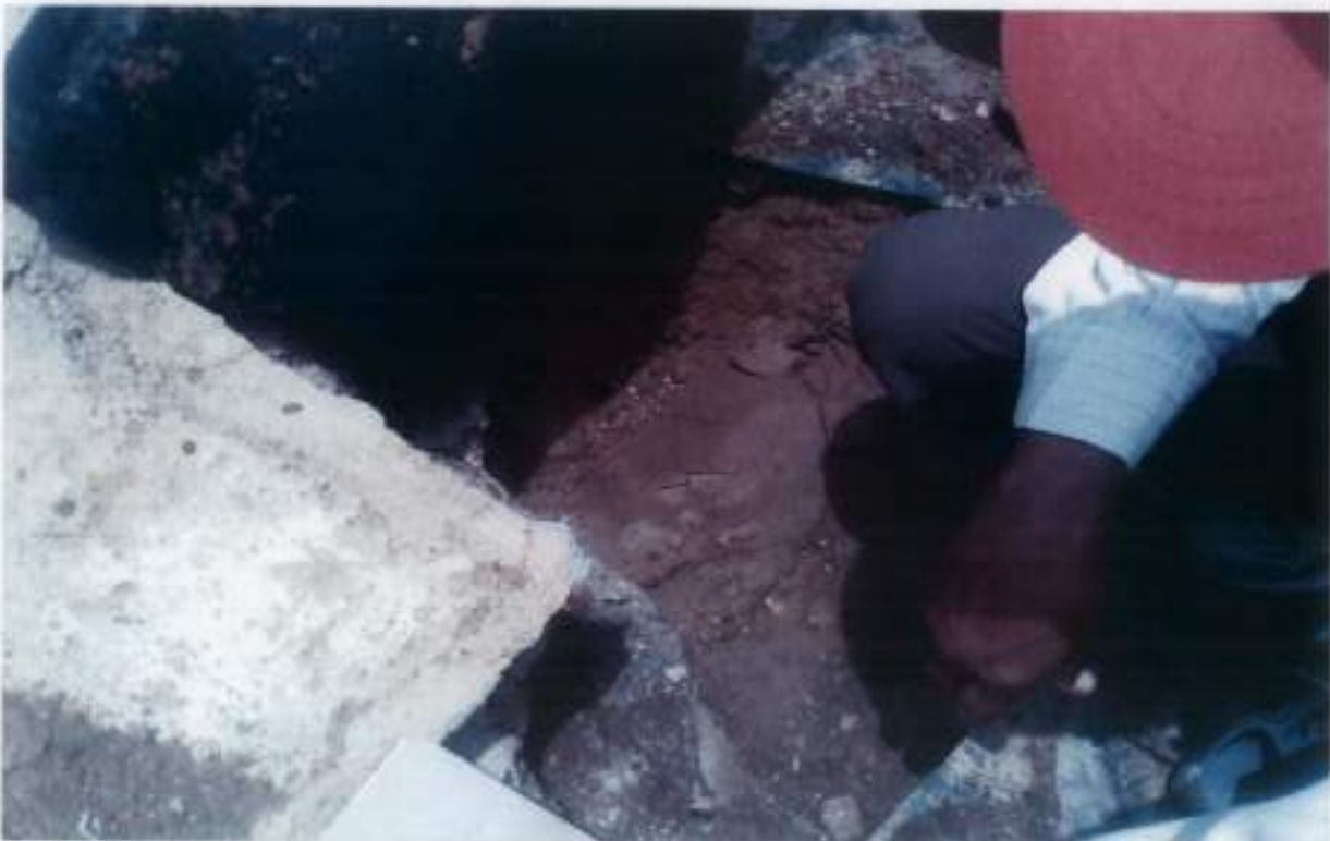
No sand layer under HDPE lining
