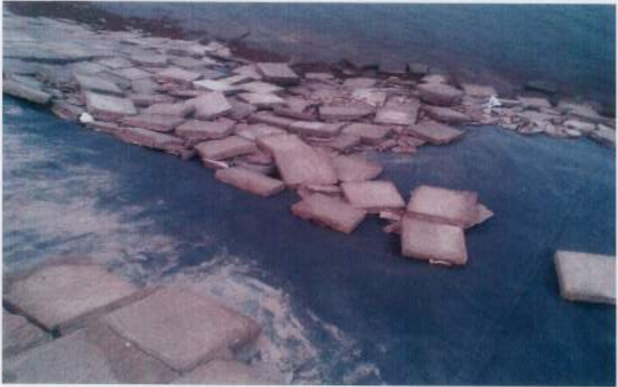
Dislodged concrete tiles on upstream slope due to subsidence
