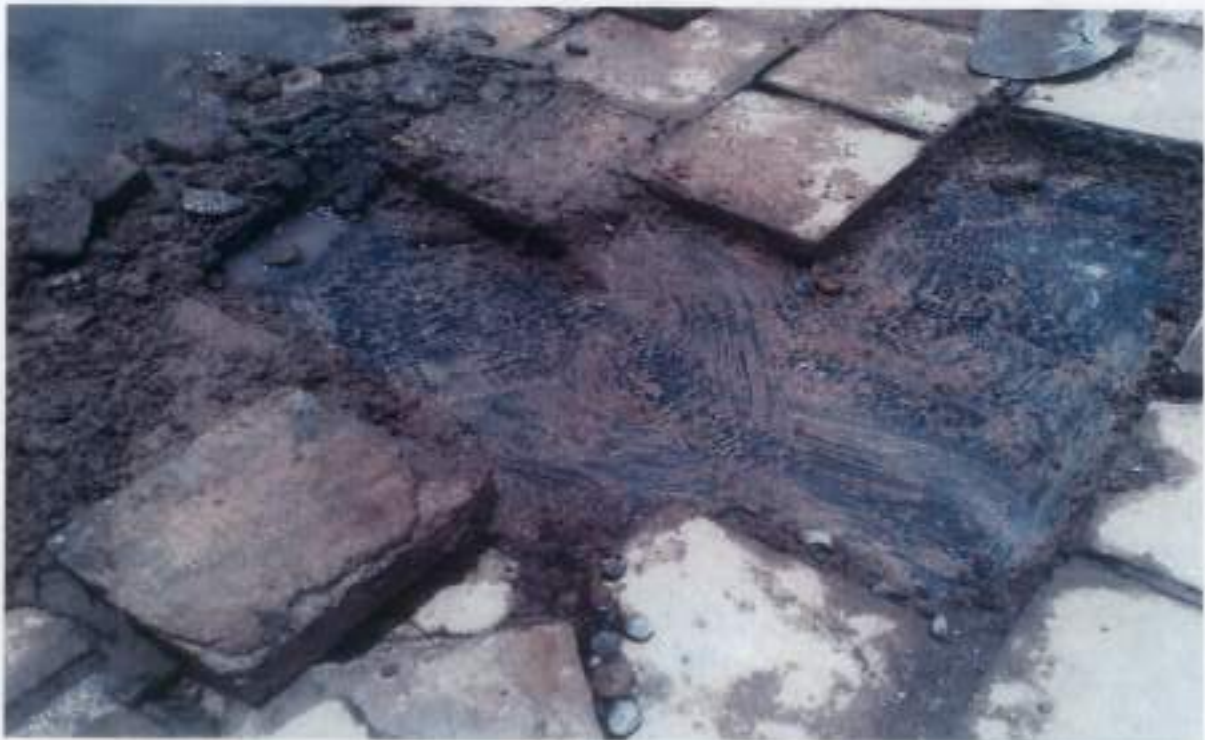
Dislodged concrete tiles at the upstream toe near the intake
